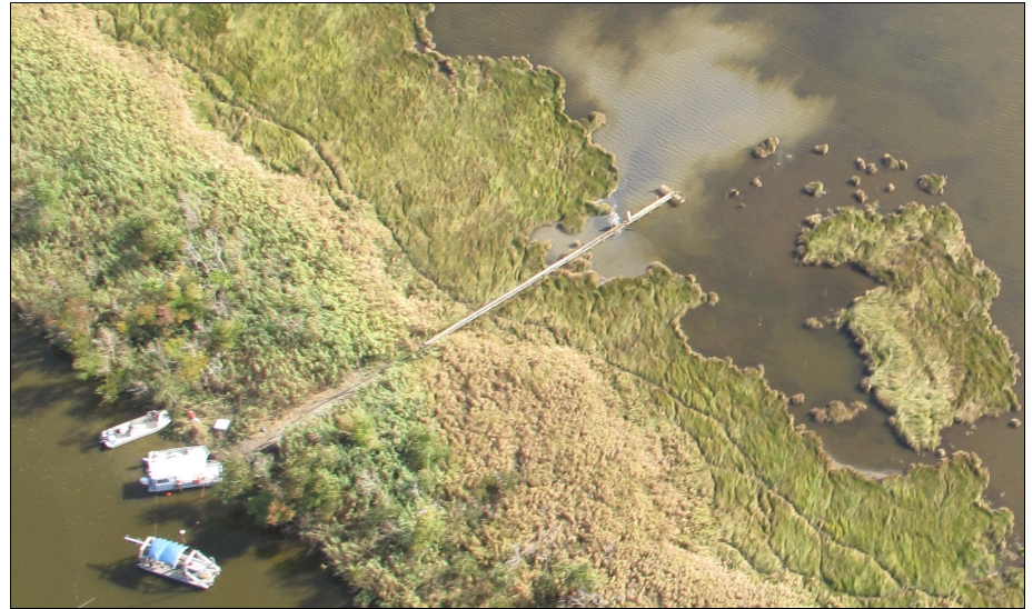
The small dredge (at the bottom of the photo) pumps mud that has settled on the bottom of the canal through a 4" hose across the spoil bank and into a pond that was created by Hurricane Ike in 2008.
